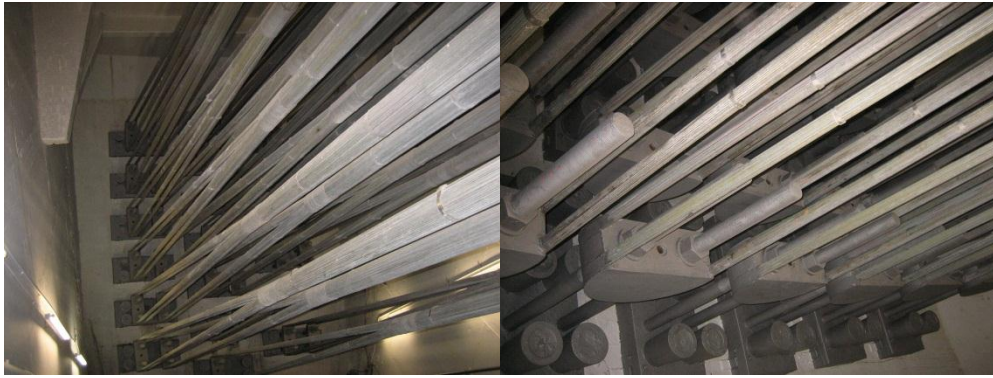
Figure 4: Inside anchorage for Forth Road Bridge showing the 19 slabs each with 6 tendons bolted to the face of the concrete tunnels
