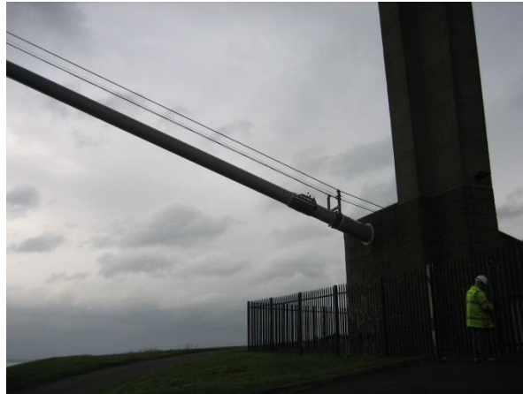
Figure 2: A suspension cable for Forth Road Bridge entering one of four anchorage chambers
