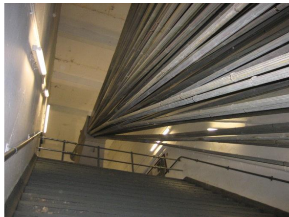
Figure 3: A suspension cable splaying as it enters anchorage chamber for Forth Road Bridge
